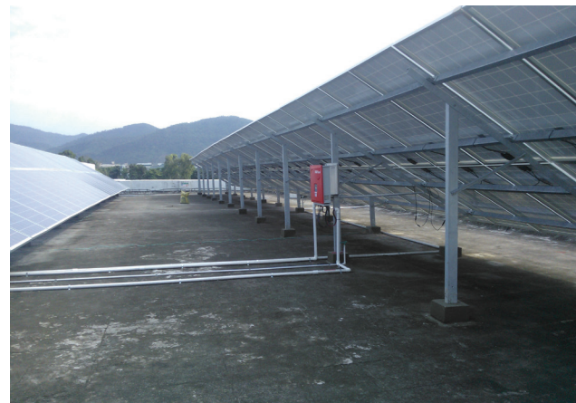
Figure 6.8: Penetrating roof mounting system
