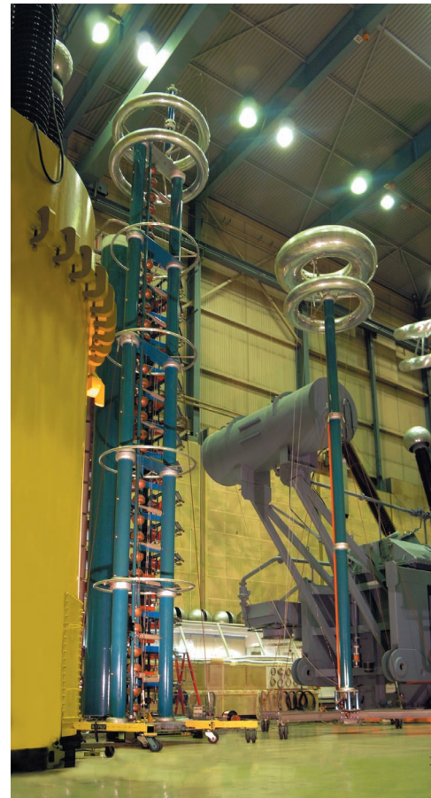
Impulse test generator and voltage divider.
