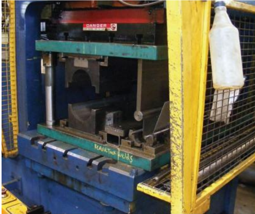
Figure 1: This 175-ton hydraulic press was severely damaged by lightning, necessitating repair or replacement of many key components, including the automation system.
